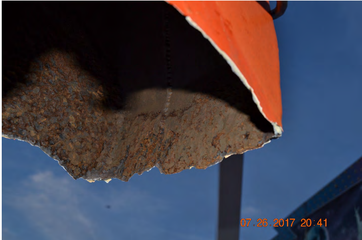
Photo #22 – Additional close up picture of the incident ride. Photo identifies the inside of the wall of metal around the arm of the broken gondola. Photograph taken by the [REDACTED] State Highway Patrol on July 26, 2017 after the incident.
