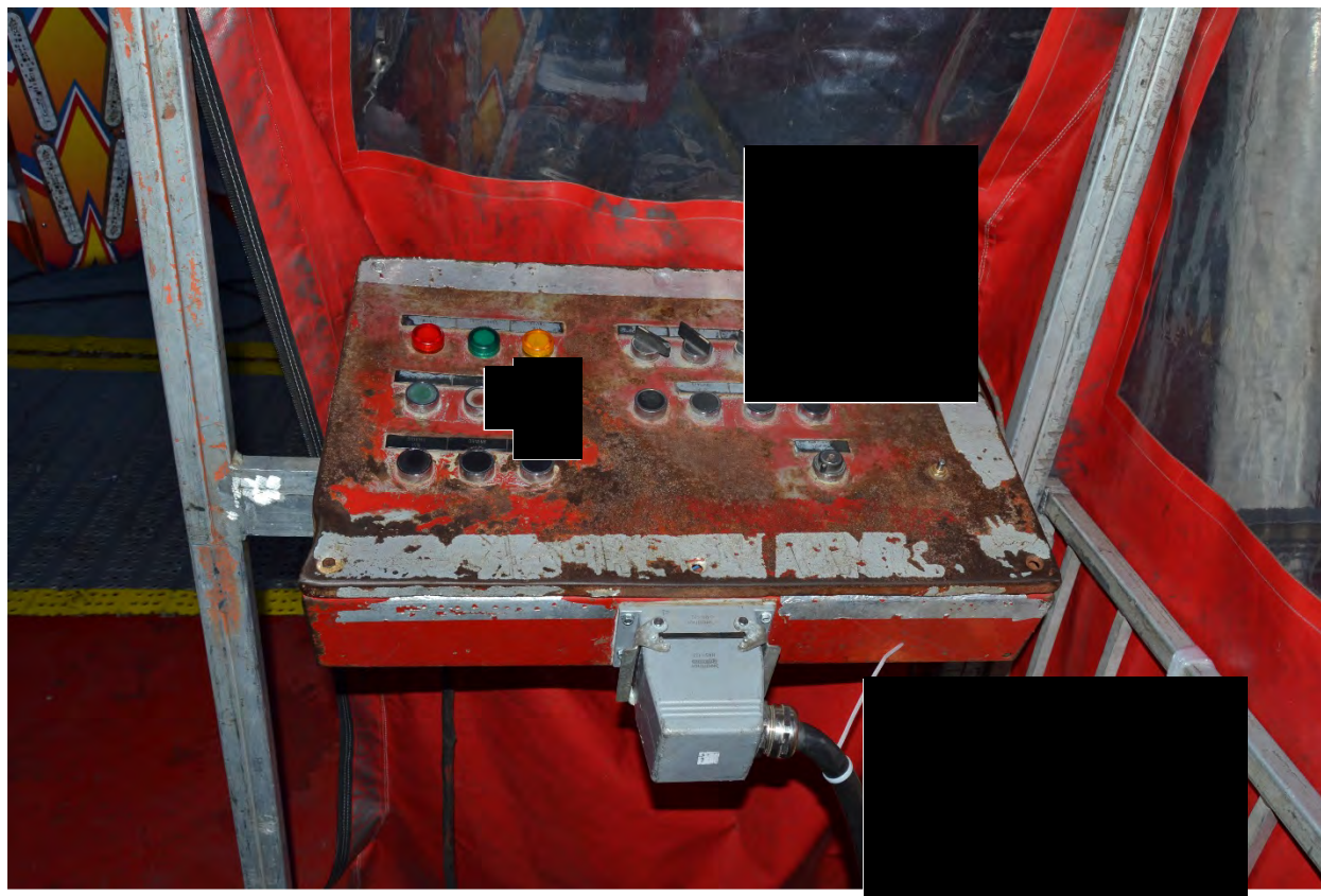
Photo #25 – Additional close up picture of the incident ride. Photo identifies the ride control panel located inside the ride control booth. Photograph taken by the [REDACTED] State Highway Patrol on July 26, 2017 after the incident.
