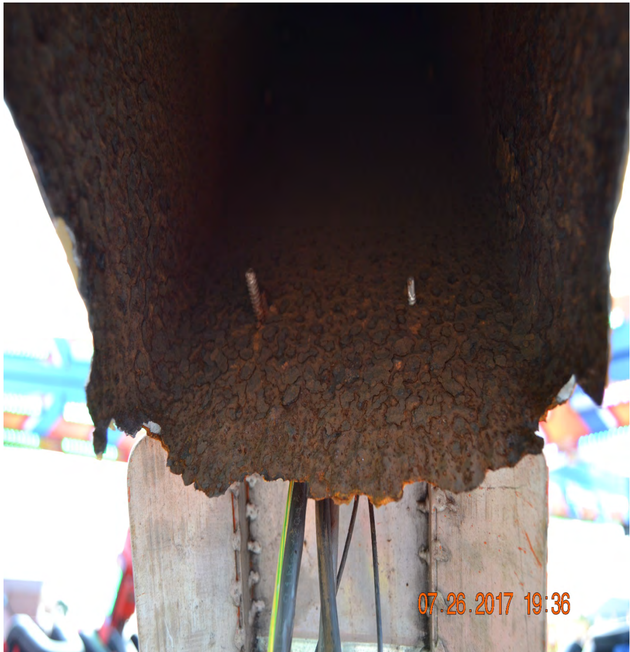
Photo #8 – Additional close up picture of the incident ride. Photo identifies the inside of the broken arm. Photograph taken by the [REDACTED] State Highway Patrol on July 26, 2017 after the incident.
