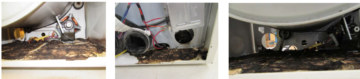
Figure 11. Base of the dryer after the test
