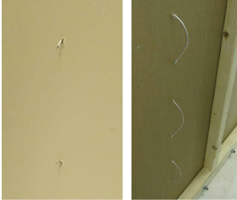
Figure 9. The image on the left shows two installed hooks from the interior of the room. The bulk of the anchor is obscured by the drywall. The image on the right shows the reverse view of three separately installed hooks.
