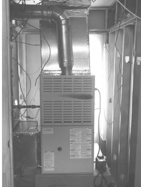
Figure 2.1. Mid-Efficiency Induced Draft Test Furnace
