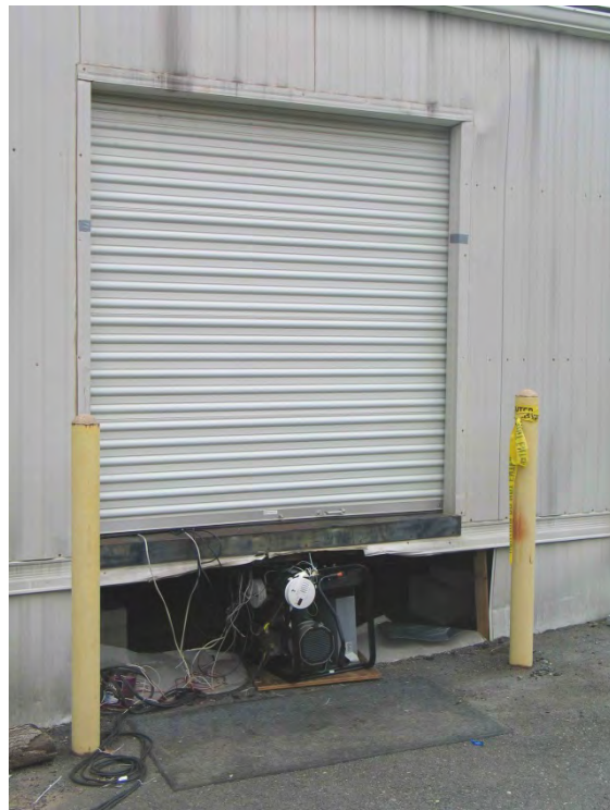
Figure A3: Outside View of the TMS Building with the Generator Placed Underneath
